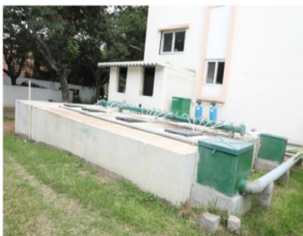
The small-scale sewage treatment plant
