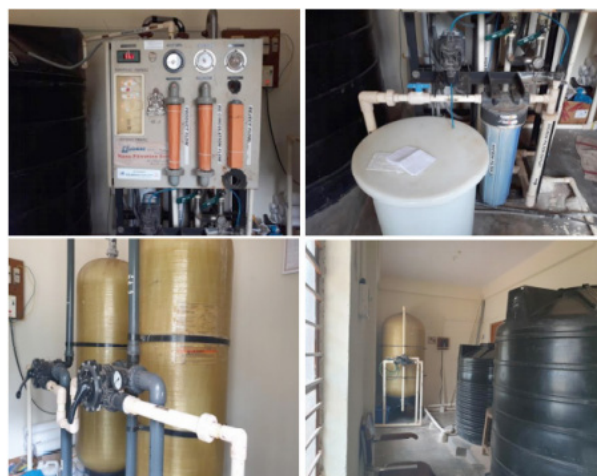
Facility for Reverse Osmosis (RO)
