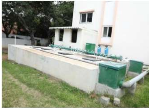
The small-scale sewage treatment plant
