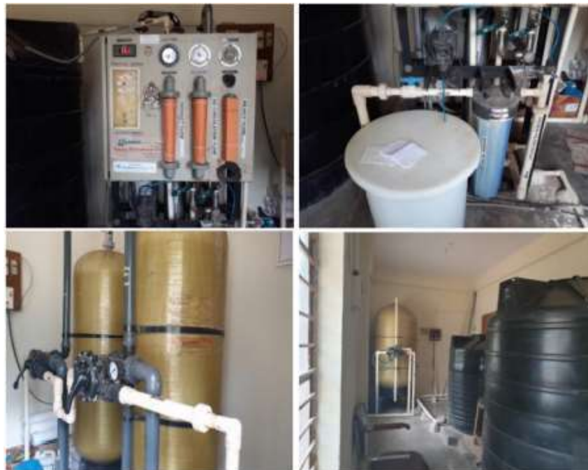
Facility for Reverse Osmosis (RO)
