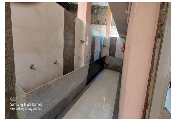
Low water release taps are installed in Hostel facilities.
