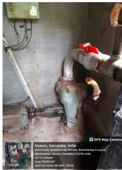
Pumps for disposing waste water into the sewage line
