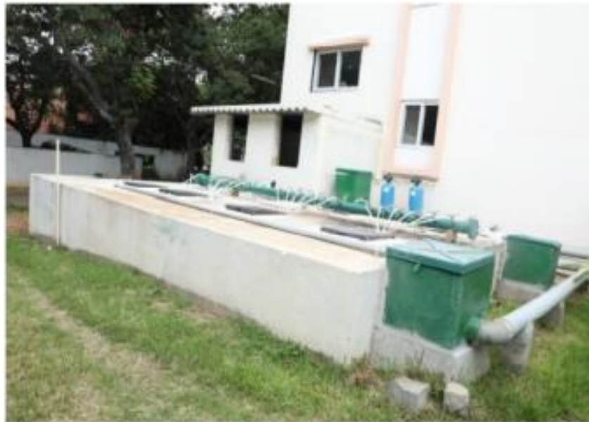
The small-scale sewage treatment plant
