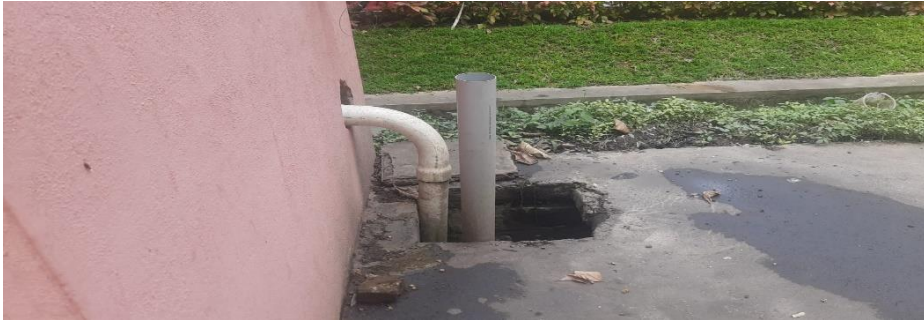
Storage tank (30,000 Litre)
