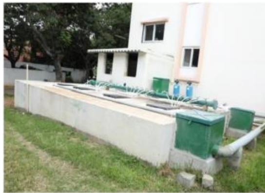
The small-scale sewage treatment plant
