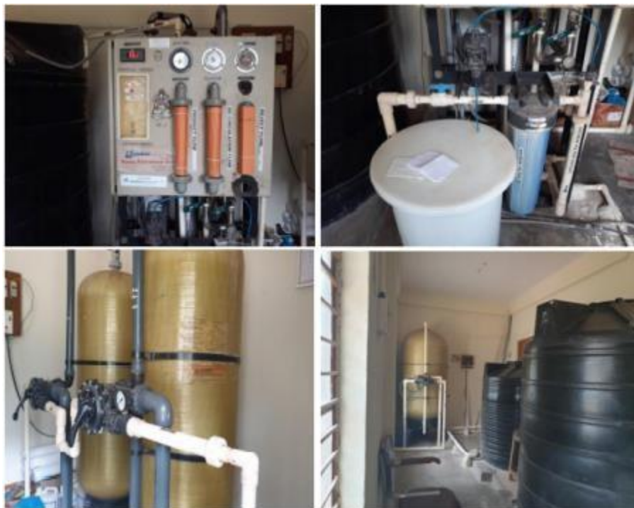
Facility for Reverse Osmosis (RO)
