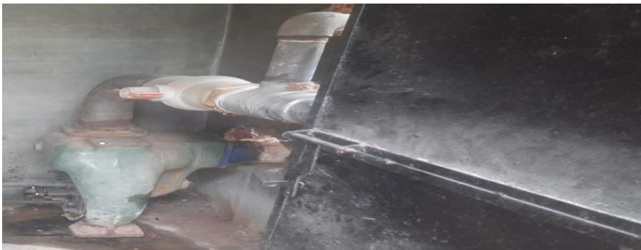
Pumps for disposing waste water into the sewage line
