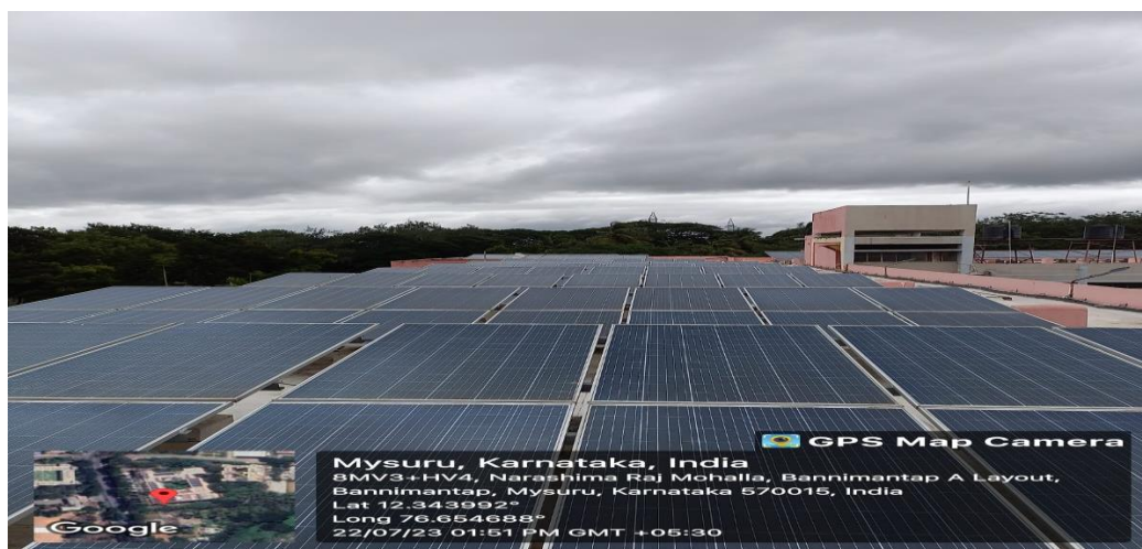
Solar panel @ JSS College of Pharmacy, Mysuru
