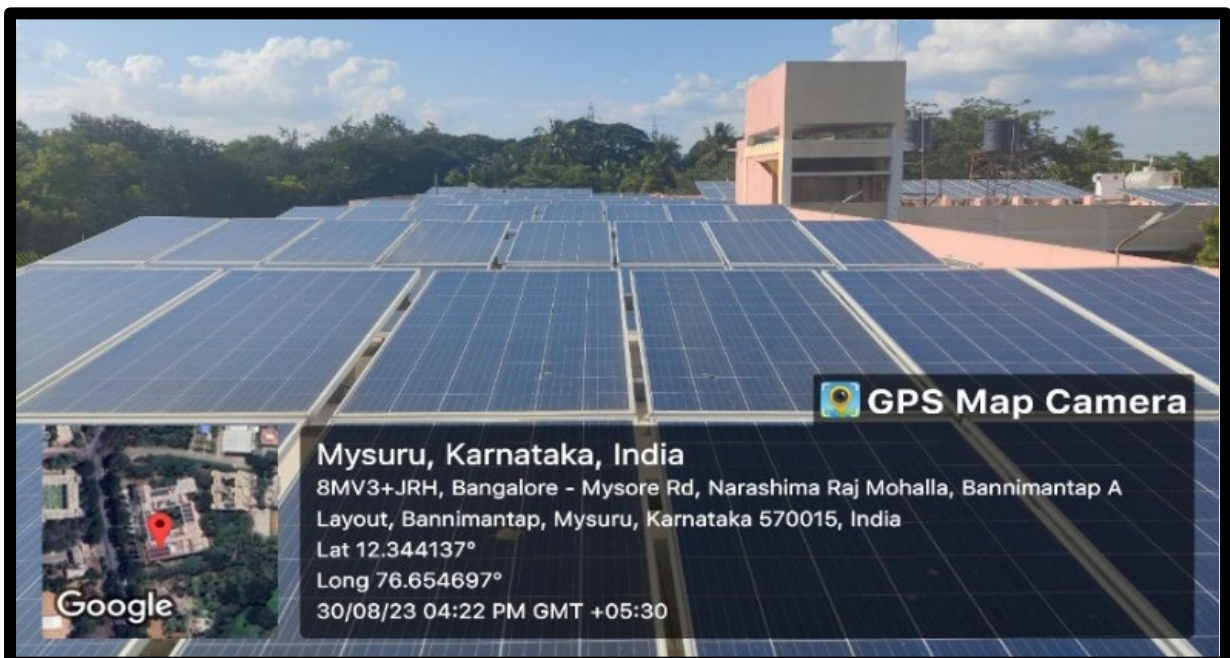
Rooftop Solar panel – JSS College of Pharmacy, Mysuru
