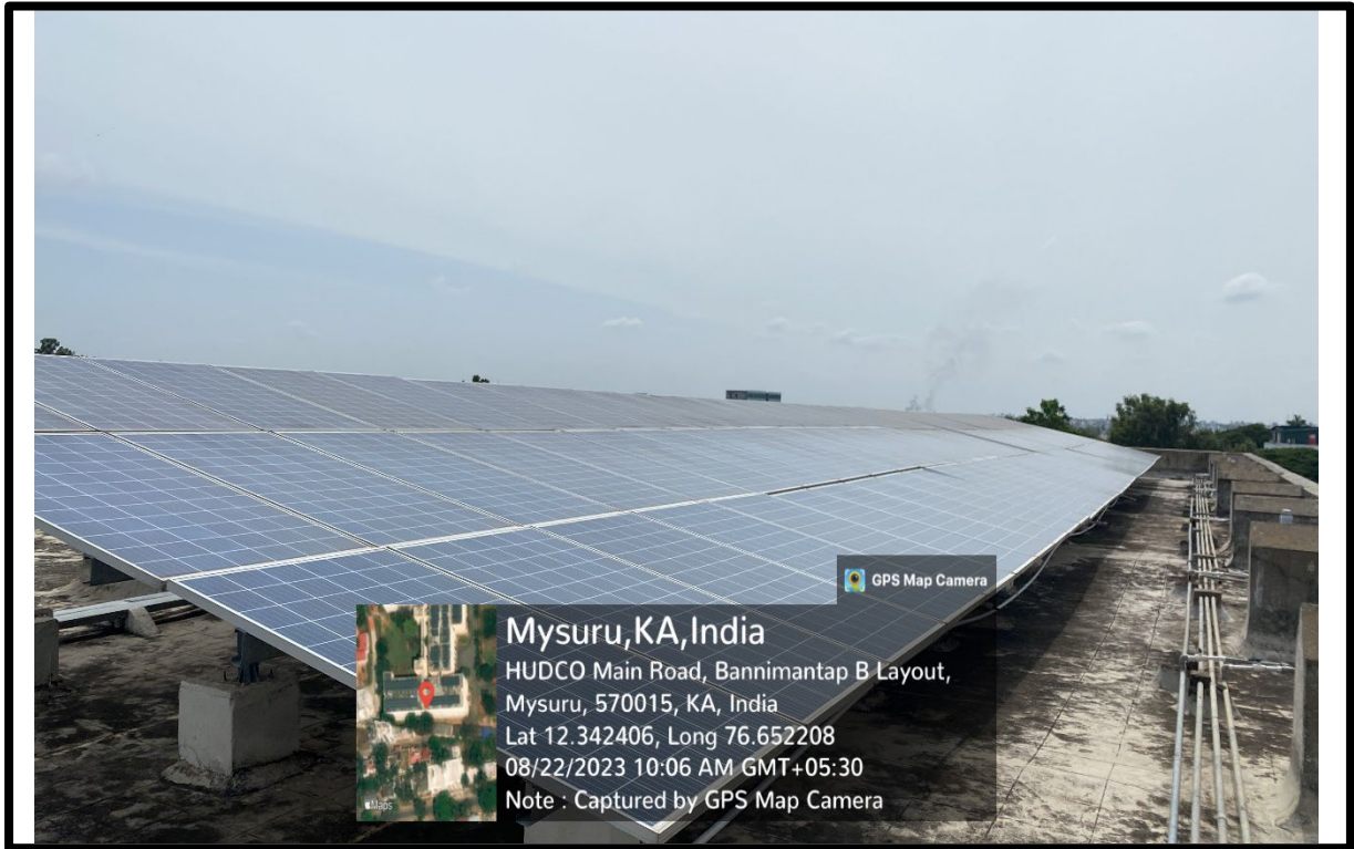
Rooftop Solar panel – JSS Dental College & Hospital, JSS AHER, Mysuru
