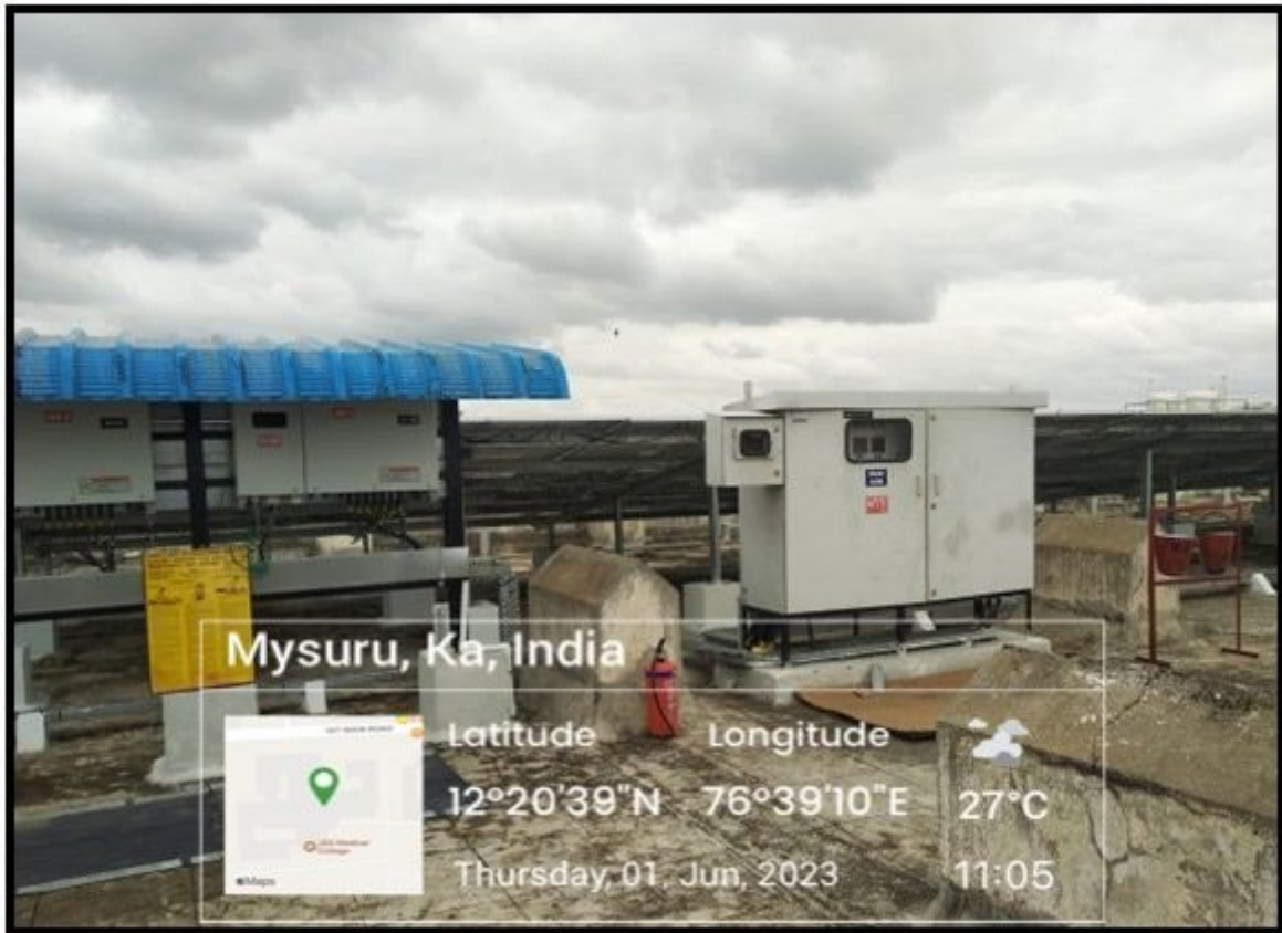
Wheeling to the grid at JSS Dental College & Hospital, JSS AHER, Mysuru
