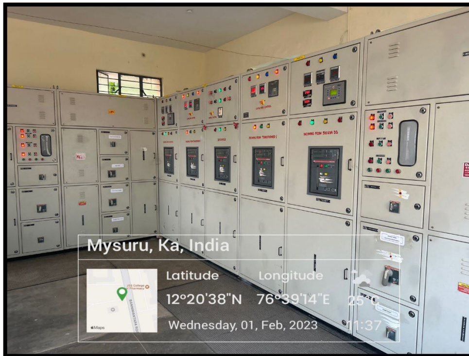
Wheeling to the grid at JSS AHER, Mysuru
