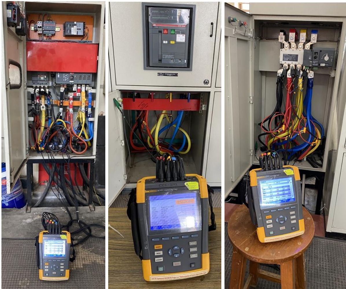
Fig 10: Incoming Supply Bus-Bar installed in the campus, JSSCPM, JSSMC, JSSCPO
