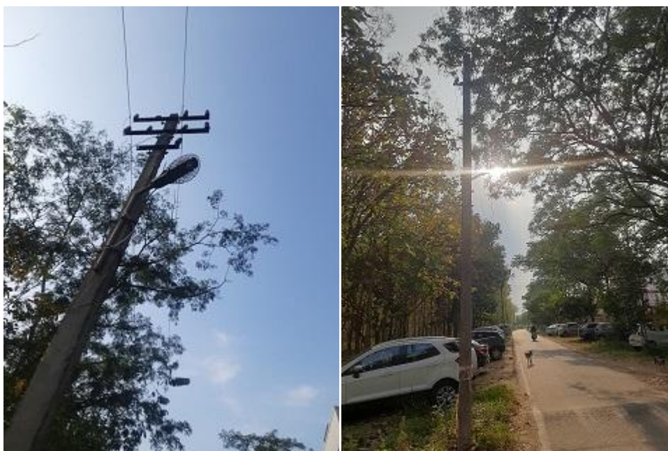
Fig 52: Trees touching the electric lines in the Medical College campus
