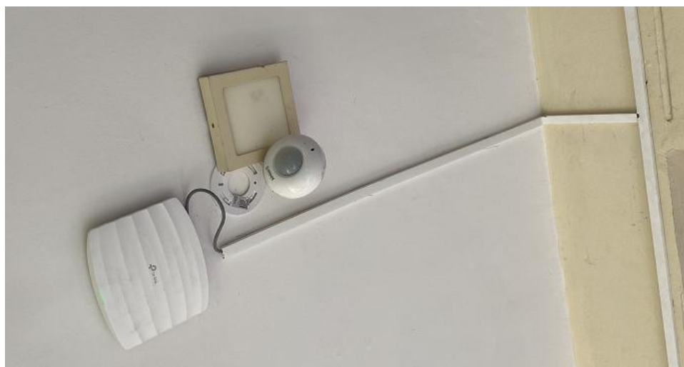
Fig 40: Occupancy / Motion Sensor in Pharmacy College Hostel, Mysuru Campus
