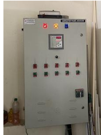
Capacitor Bank Panel in Pharmacy College, Mysuru
