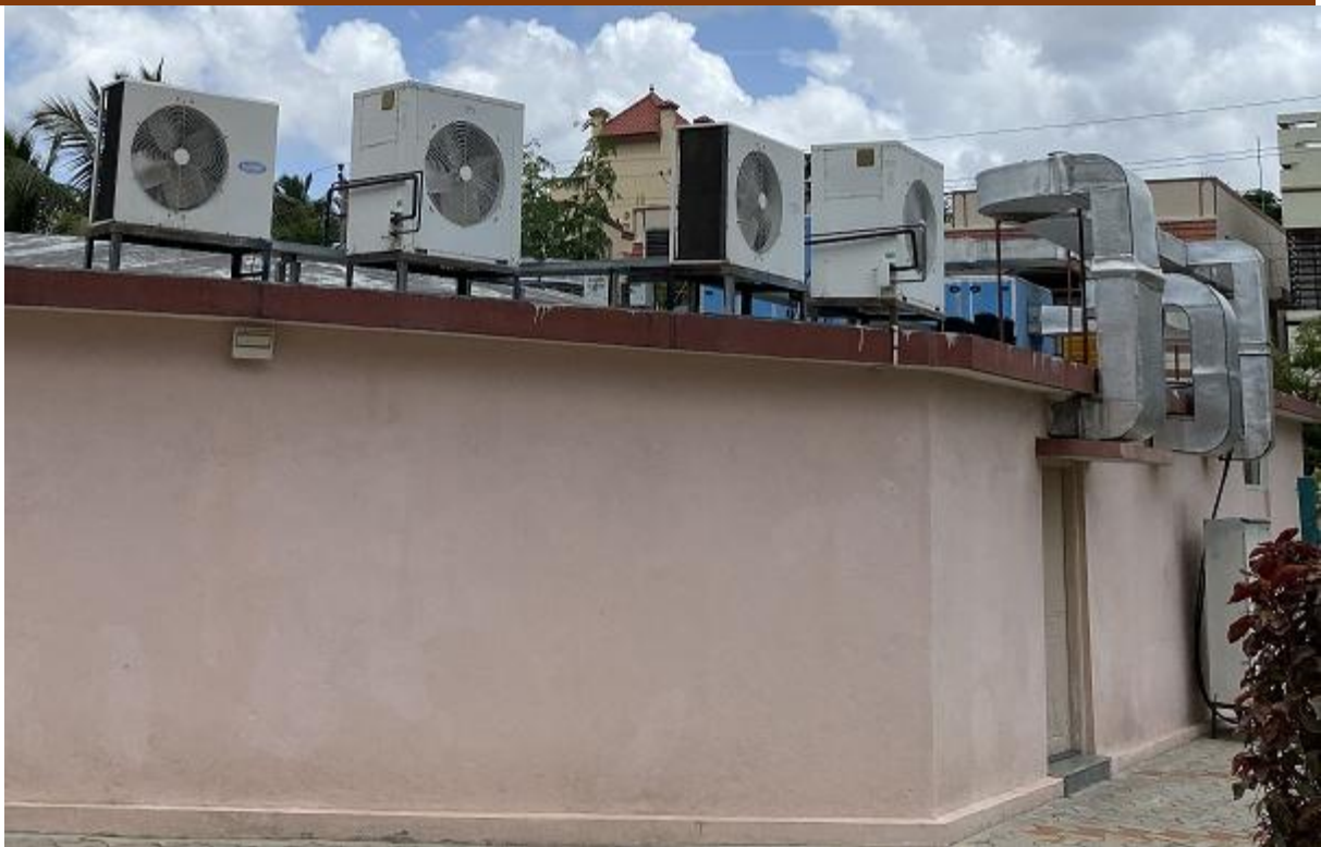
Fig 47: Existing Air Conditioners in the facility that can be fitted with VFD
