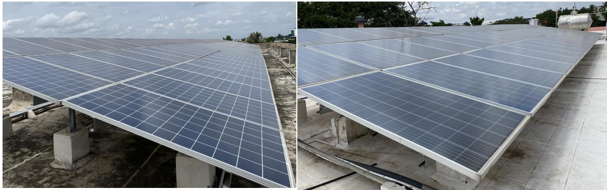
Fig 6: Shows Solar Panels installed at Left: Dental College, Right: Pharmacy College, Mysuru
