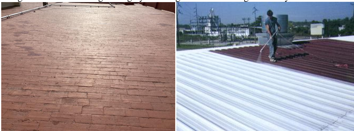
Fig 49: Existing Roof in Ramanuja Road Building and Proposed white paint for the roof
