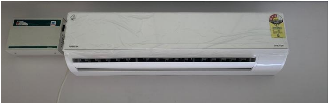
Fig 38: New Inverter AC in the campus
