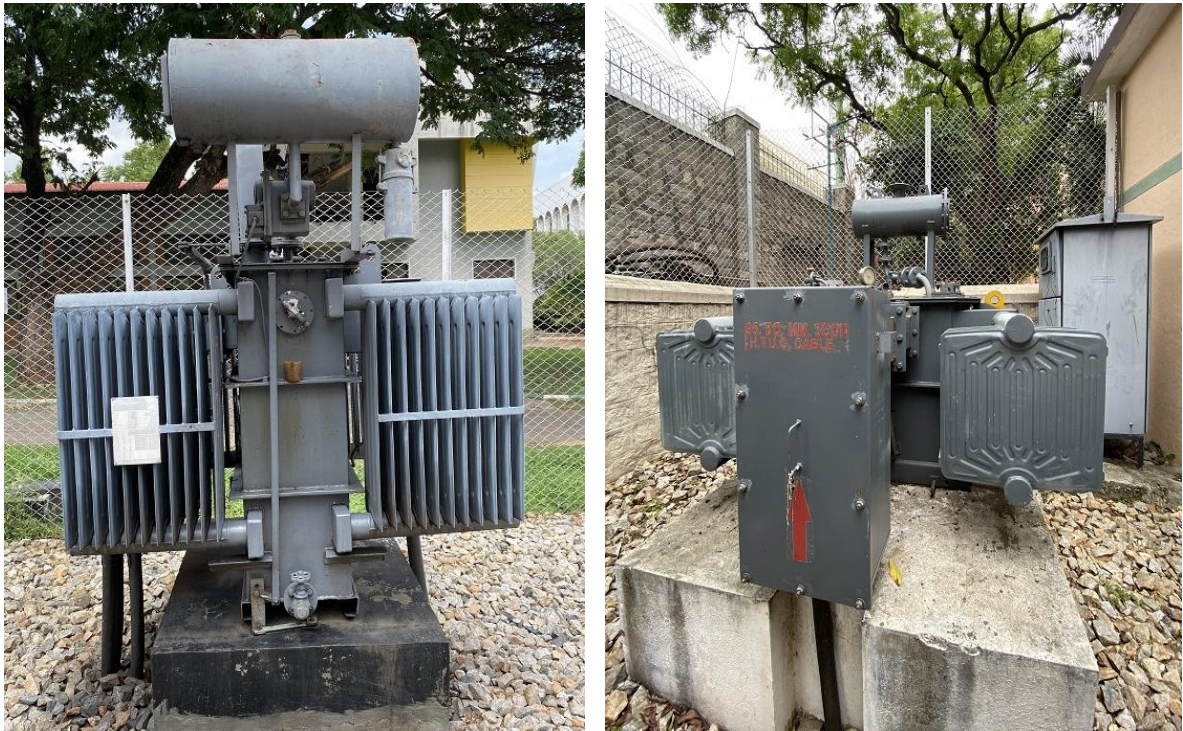
Fig 4: Transformers installed for incoming supply in Medical College and Pharmacy College
