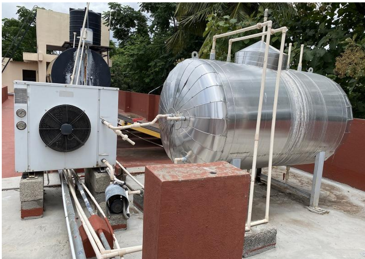
Fig 42: Existing Heat pump in Pharmacy Hostel
