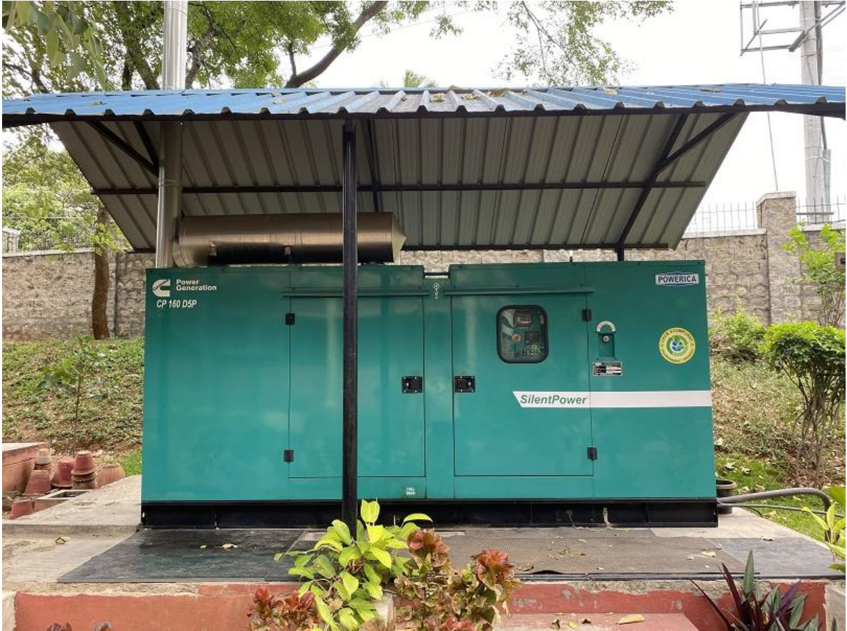
Fig 21: 160kVA Diesel Generator installed at the College of Pharmacy, Mysuru Campus
