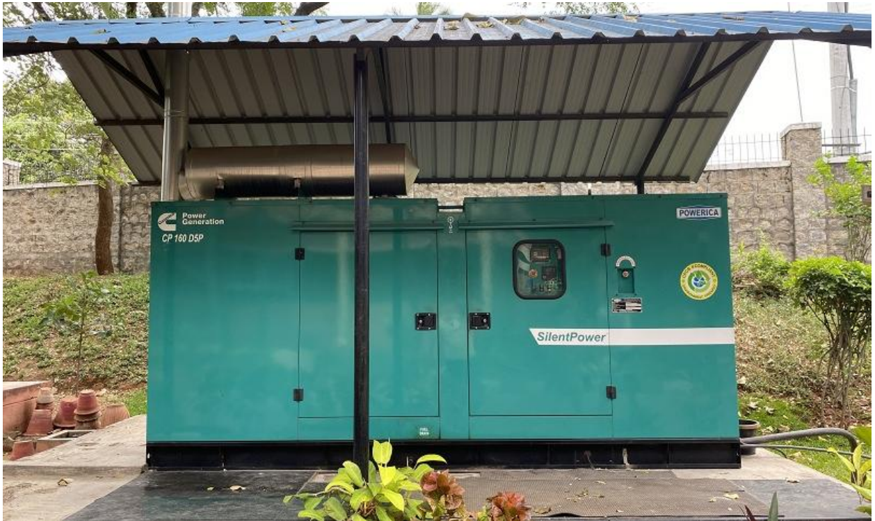
Fig 8: 160kVA Diesel Generator installed at the College of Pharmacy, Mysuru Campus
