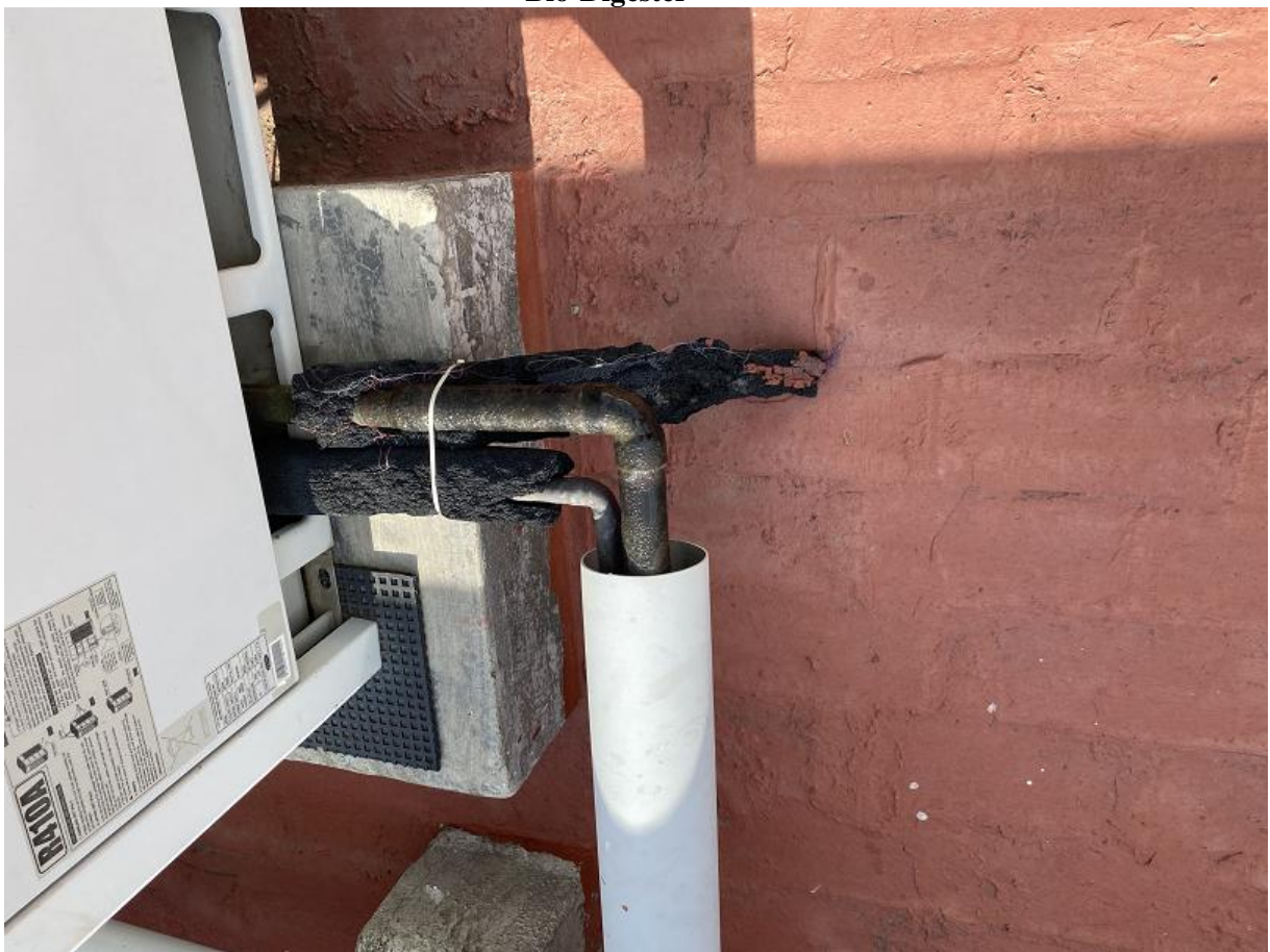
Fig 59: Torn Insulation on 50 Ton AC in JSS Ramanuja Road Campus, Mysuru
