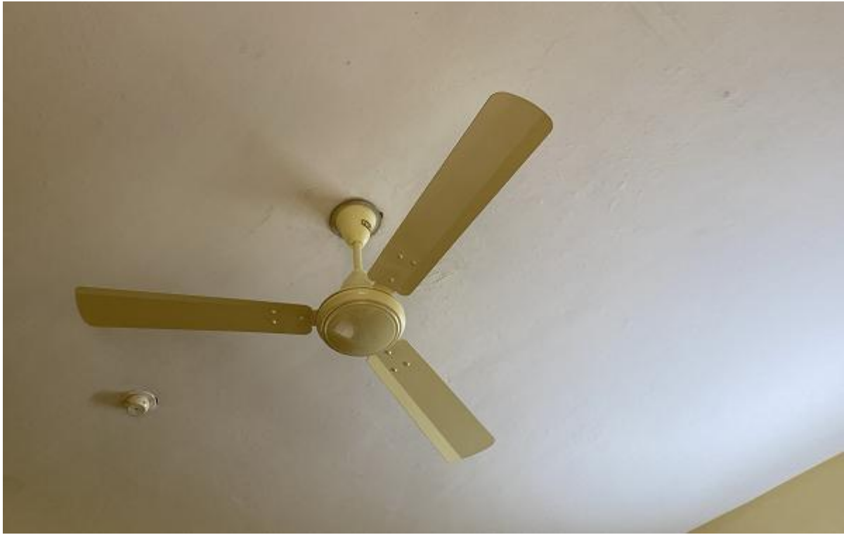
Fig 34: BLDC Fan in JSS College of Pharmacy Hostel, Mysuru Campus
