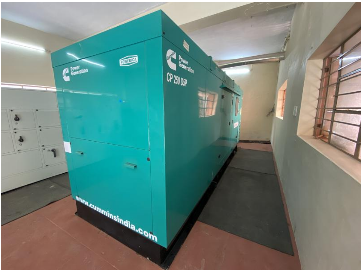
Fig 9: 250 kVA Diesel Generator installed at the Pharmacy, Ooty Campus
