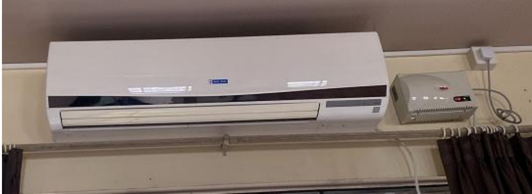
Fig 37: Old Non-inverter AC in the campus
