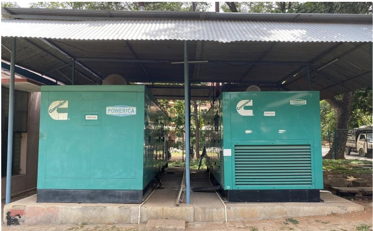
Fig 7: Diesel Generators (500 kVA & 380kVA) installed at the Medical College Campus
