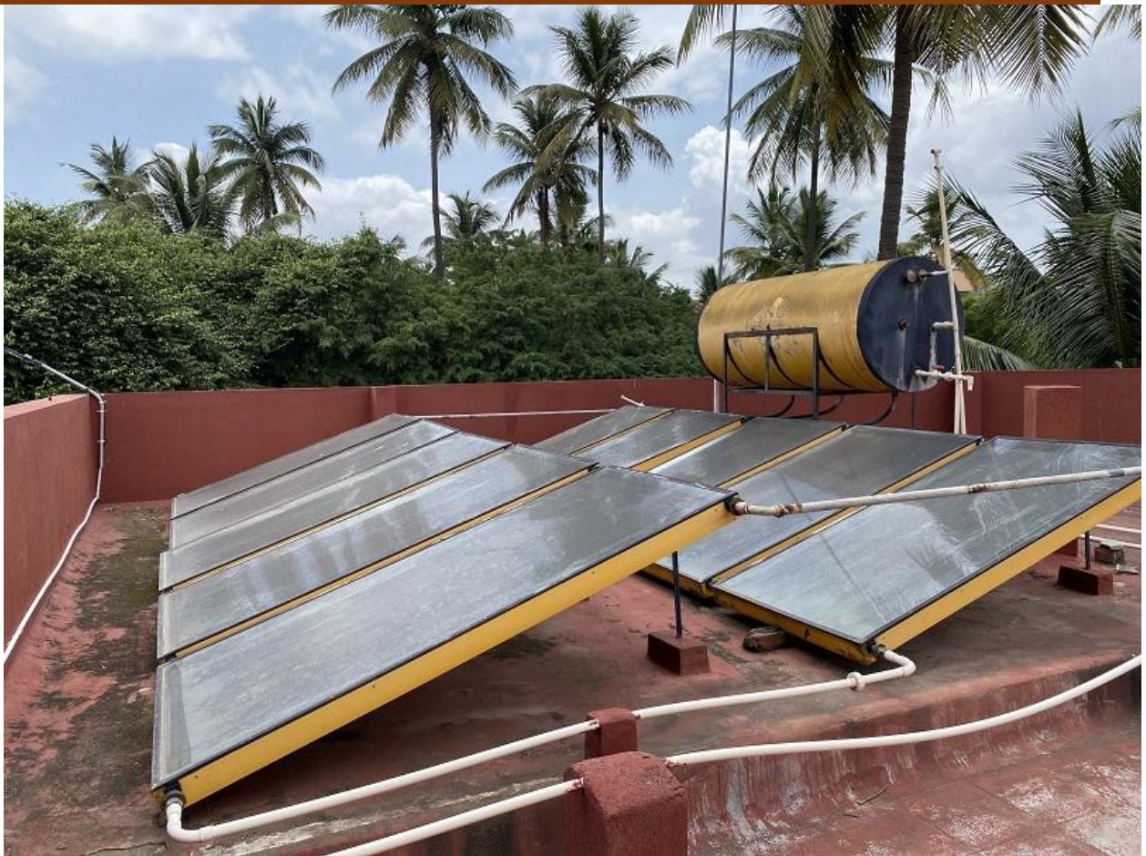
Fig 43: Disconnected Solar Water Heater in Pharmacy Hostel
