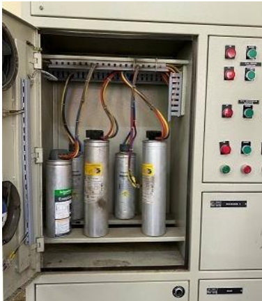
Capacitor Bank in Medical College
