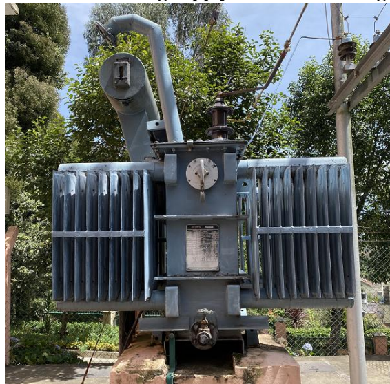
Fig 5: Transformers installed for incoming supply at JSS College of Pharmacy, Ooty
