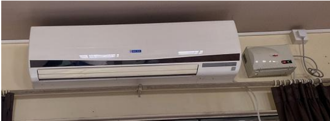
Fig 37: Old Non-inverter AC in the campus
