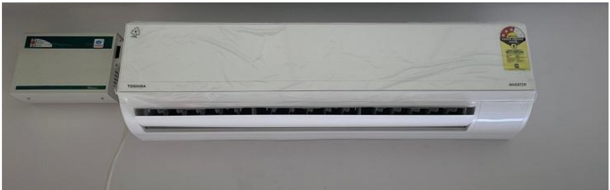
Fig 38: New Inverter AC in the campus
