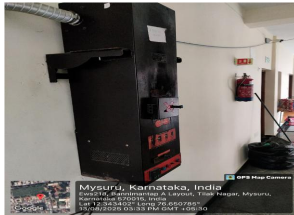
Sanitary napkin Incinerator
