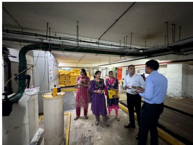
Inspection of process of chlorination and functioning of the pump
