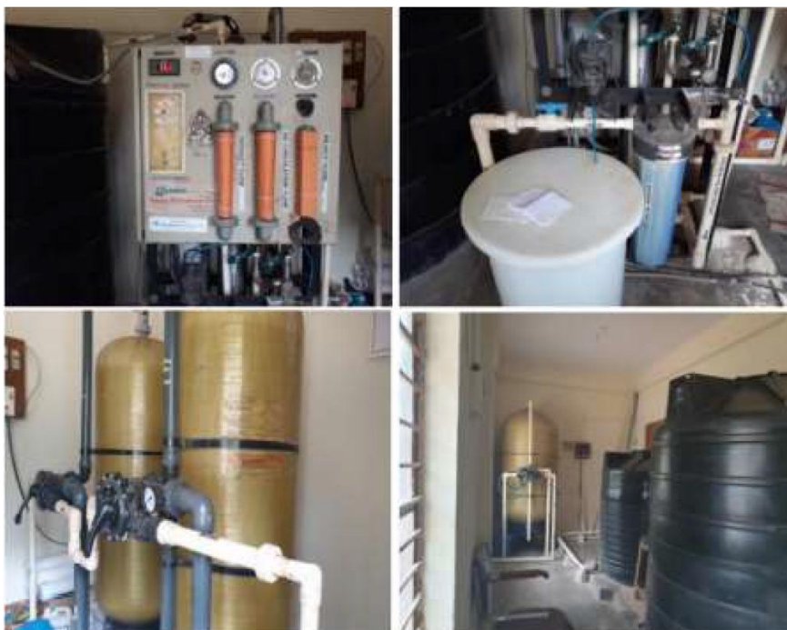
Facility for Reverse Osmosis (RO)
