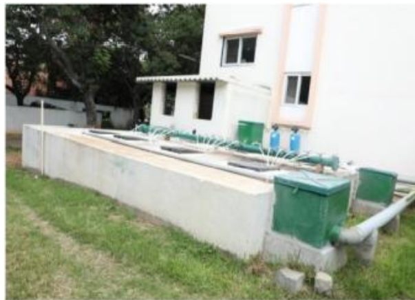
The small-scale sewage treatment plant
