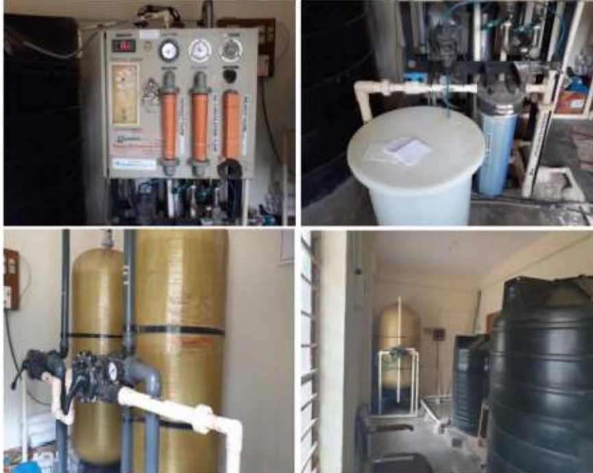
Facility for Reverse Osmosis (RO)
